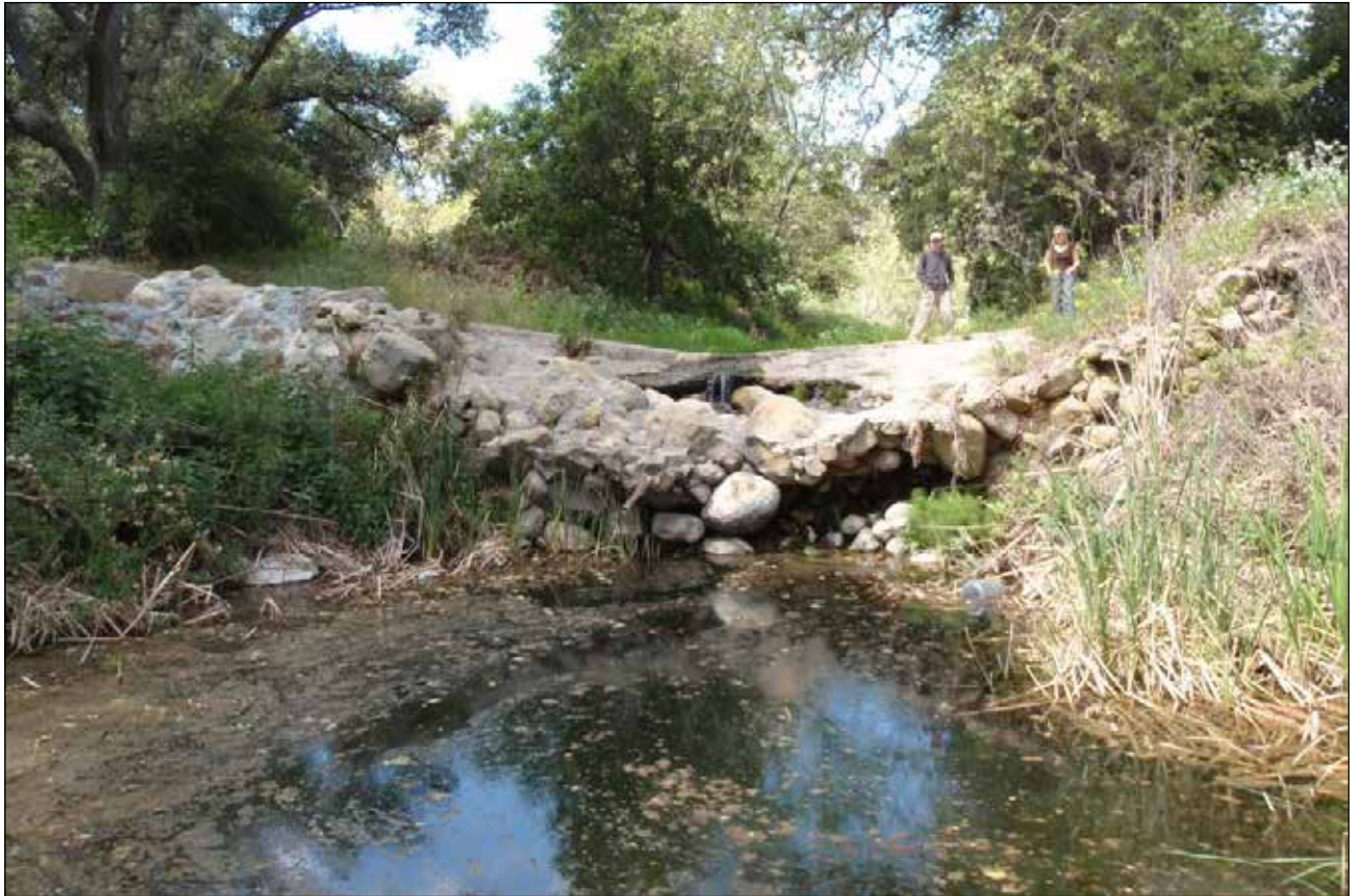
This low-flow crossing on Tajiguas Creek was a barrier to fish before work was begun.
